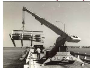
Most of the original bridges had catwalks on at least one side of the bridge for fishing even the 7-Mile Bridge. They were removed in the 1980's when construction of the new bridges began.
